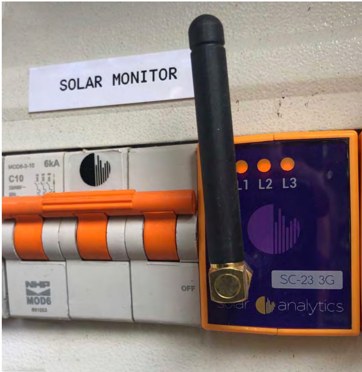
A consumption monitor in my switchboard.
