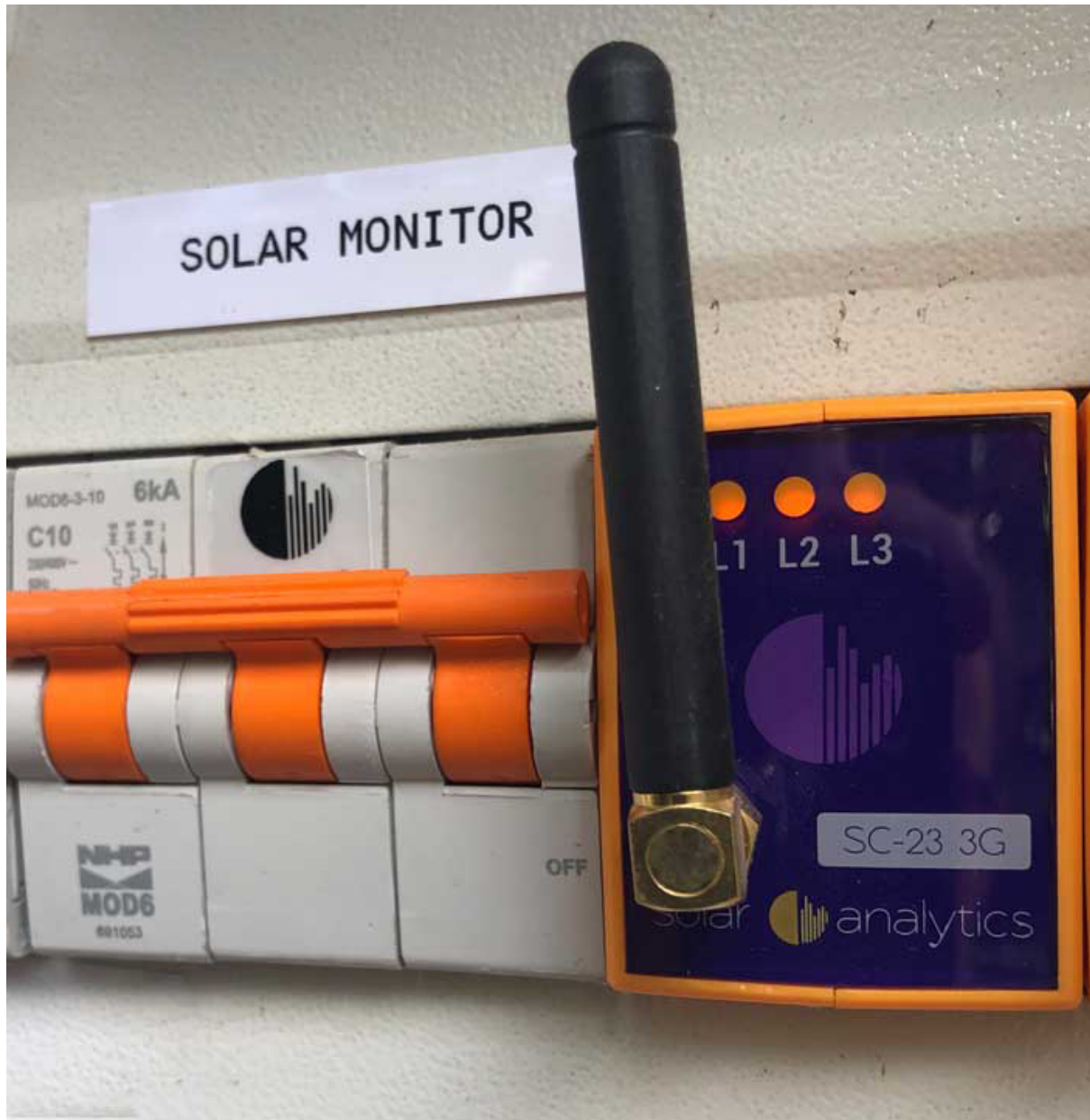
A consumption monitor in my switchboard.
