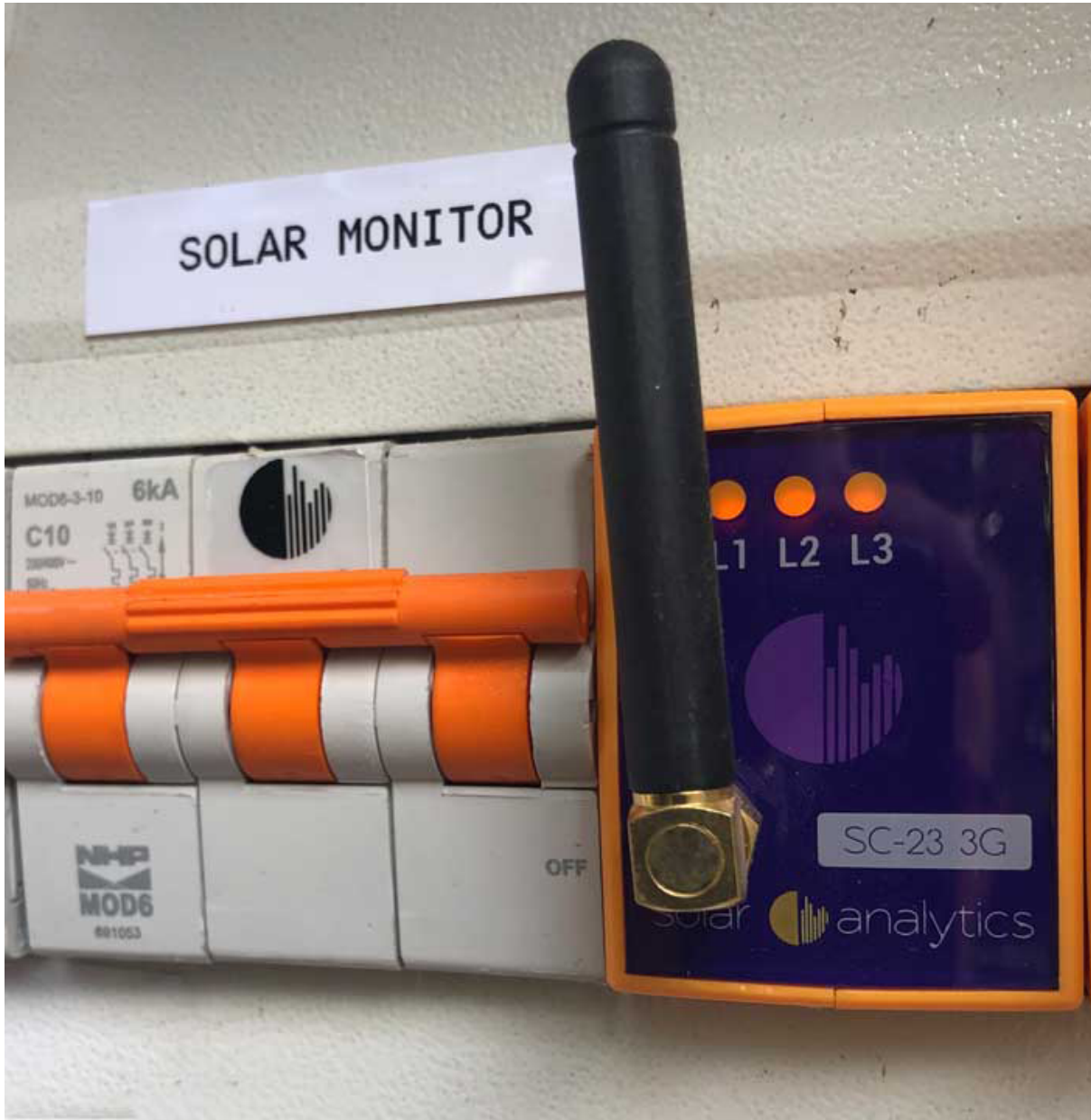
A consumption monitor in my switchboard.
